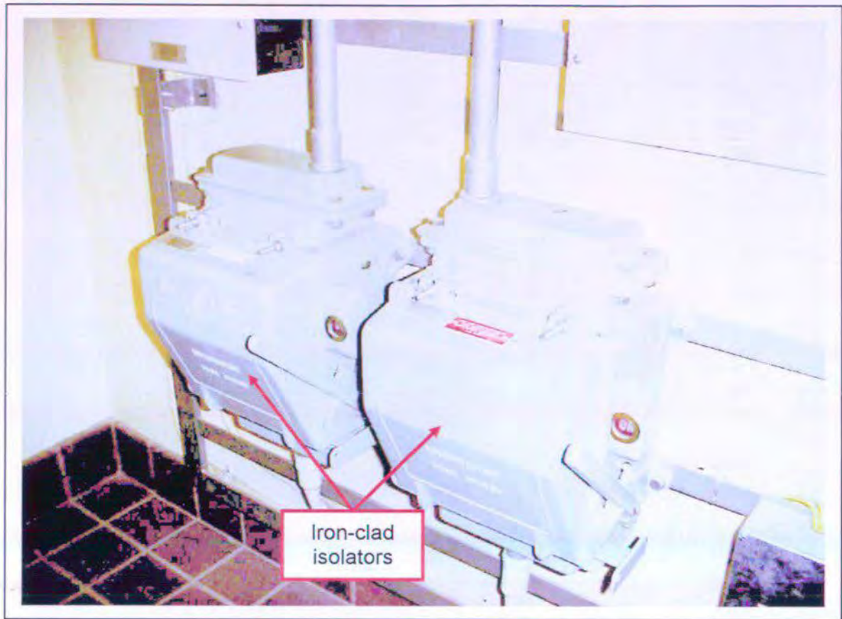
Figure 13: Material Strongly presumed To Contain Asbestos
