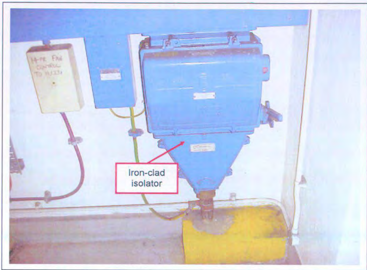
Figure 16: Material Strongly presumed To Contain Asbestos
