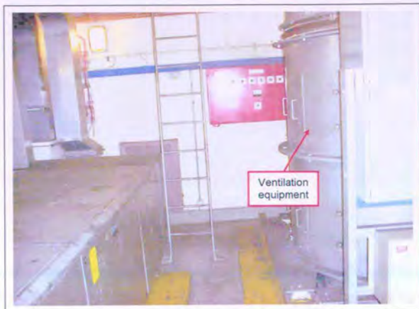
Figure 17: Material Strongly presumed To Contain Asbestos
